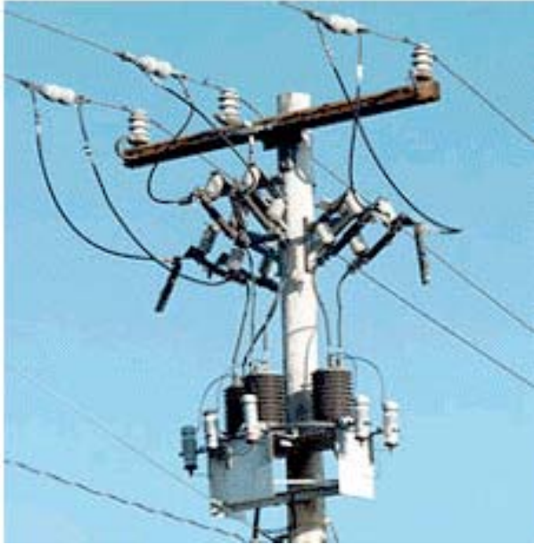
A transformer on a utility pole.
