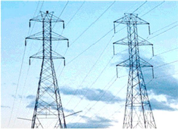
Power transmission lines.
