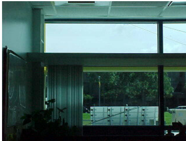
Lightshelves in the South facing windows at FSEC
