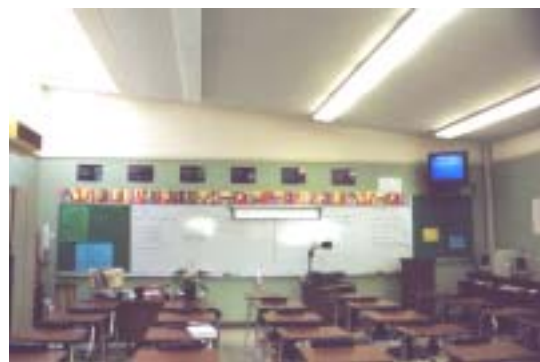
Lighting Controls, Oakridge High School: Automatic photosensor controls turn off first bank of lights next to skylight well. The light fixtures are arranged parallel to skylights to left and windows (out of picture) to right, while whiteboard is located perpendicular to windows and skylights. Photo courtesy Lisa Heschong
