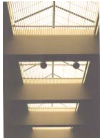
Linear skylight in multipurpose room includes electrically operated louvers to reduce brightness when needed. Photo courtesy Lisa Heschong.
