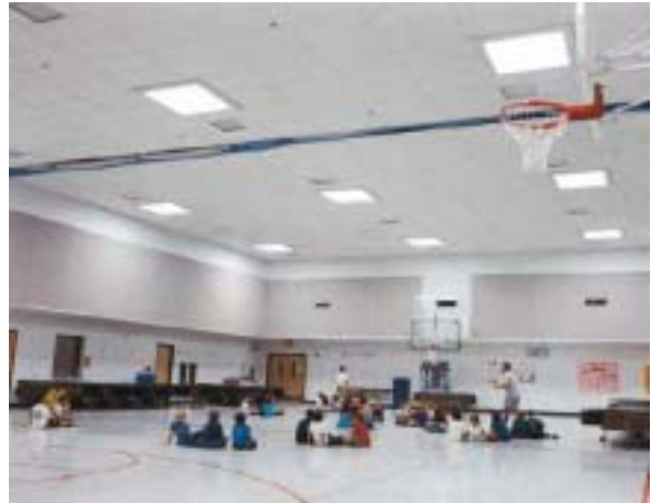
Grid of skylights in Peoria Gymnasium provide even illumination across the space. Photo courtesy Natural Lighting Co., Inc.
