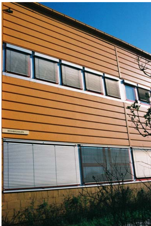
Figure 8: Reflective Venetian blinds at a building at Luleå University of Technology.
