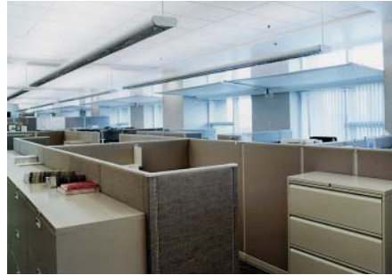
Interior lightshelves increase the ambient daylight into the office, and block the sun.
