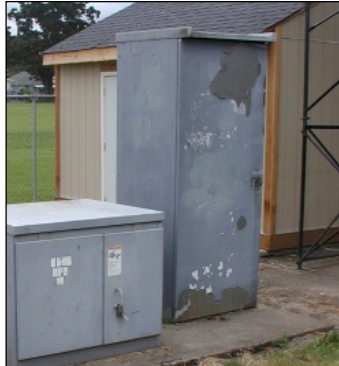
Poor Paint Finish
